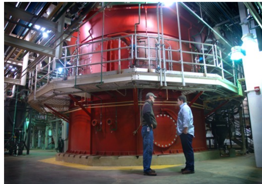
Wastewater solids (SSI) incinerator, St. Paul, MN
