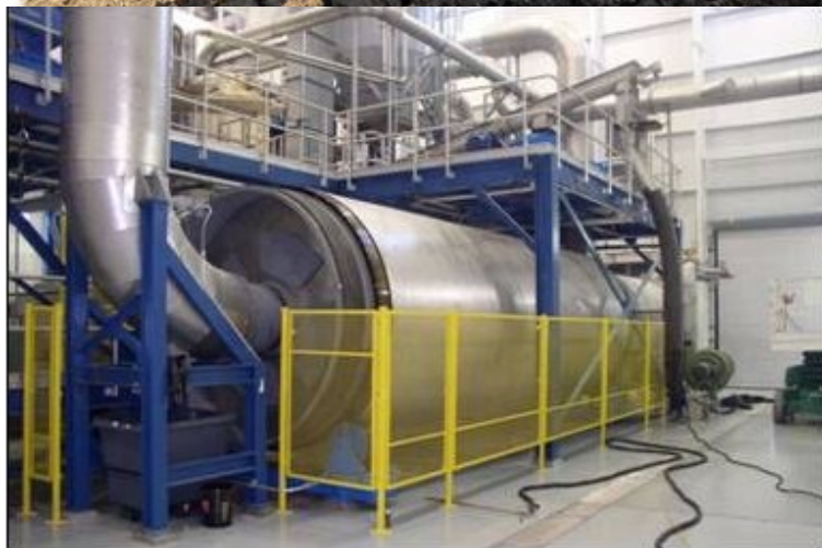
Rotary drum dryer, South Cary, NC
